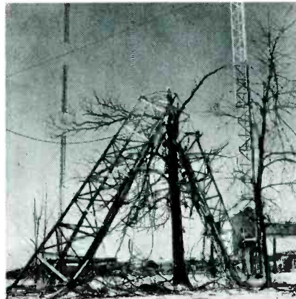
Fig. 1. Top section fell from front tower.
