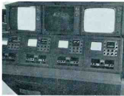
Fig. 4. Camera control units and monitors.
