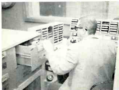
Fig. 1. Cartridge machines mounted on drawer slides to facilitate maintenance.
