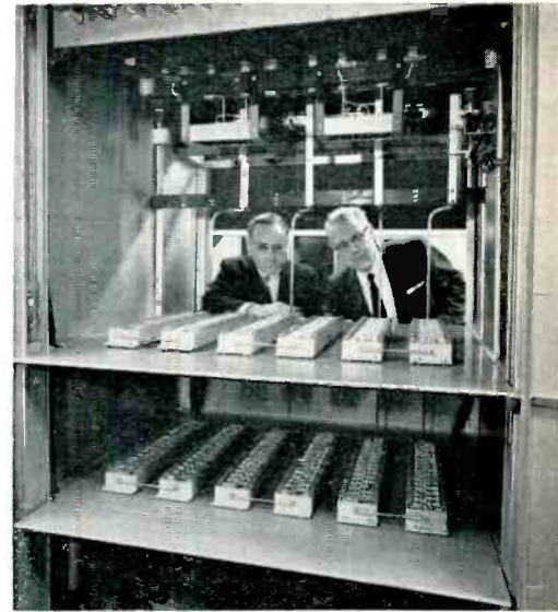
Fig. 2. Twenty-six silicon rectifier stacks in this cabinet supply high and low voltage.
