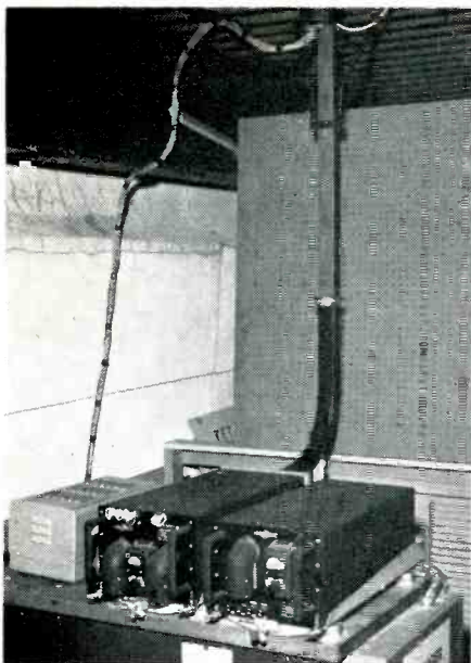
Figure 9 RT Unit, Synchronizer and Junction Box.
