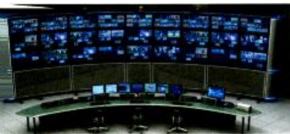
Using multiviewers, the MCR now more resembles a NOC, displaying the screens of playout servers, network traffic and more.
