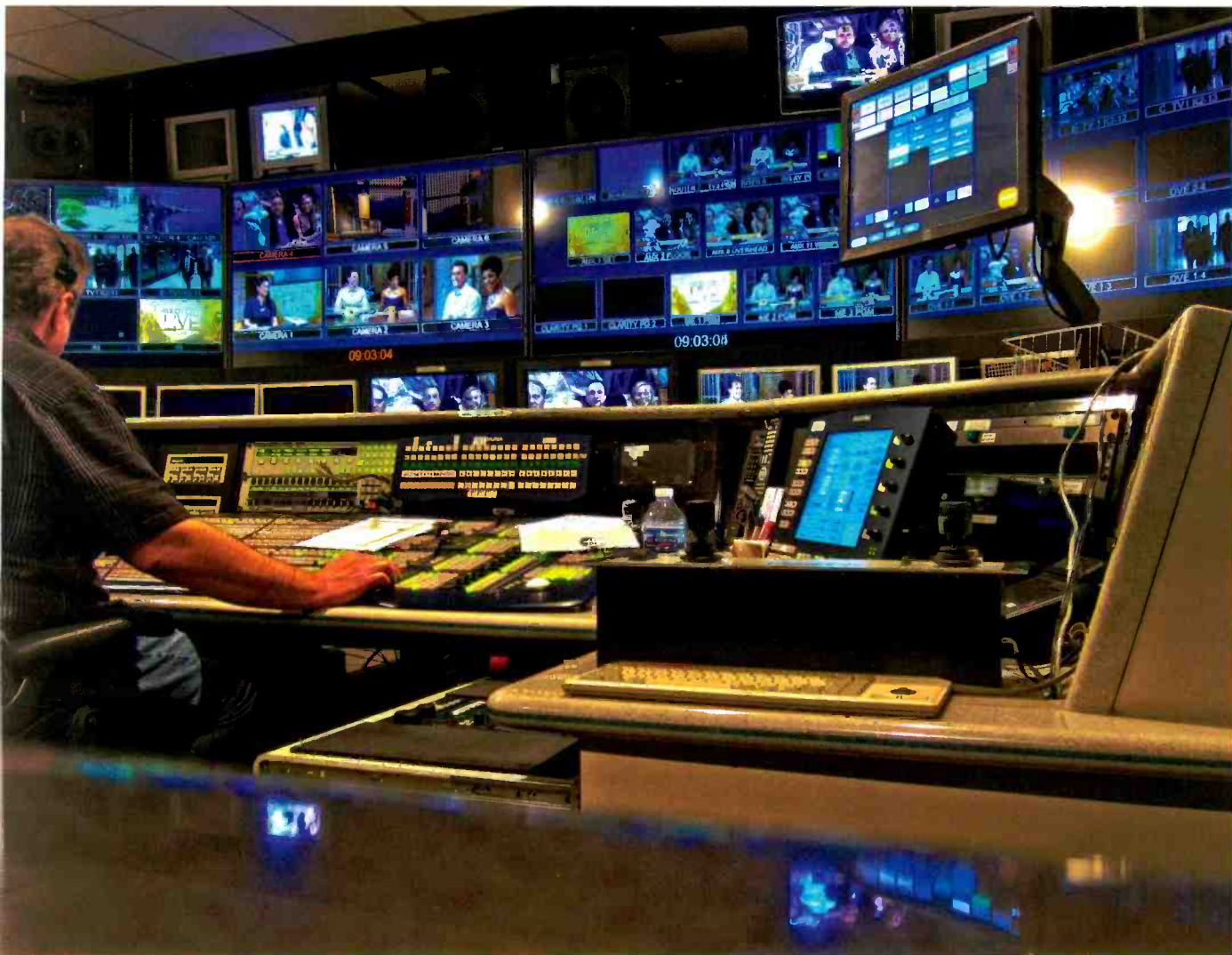
TV 1, WLS-TV's main control room, was designed around a Snell Kahuna 4ME production switcher and was already HD-capable. A Genelec 5.1 monitoring system continues to serve the control room. Photo courtesy Thomas Hebel.
