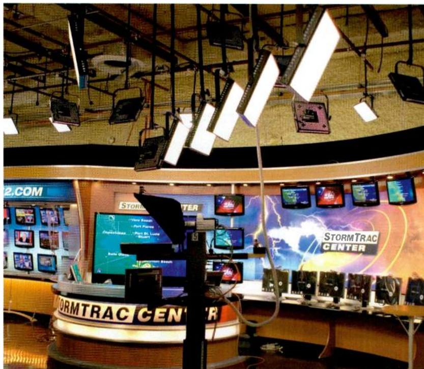
WPEC-TV in West Palm Beach, CA, recently became the first studio to light its entire news studio with LED fixtures from Litepanels. The station now draws only 3kW with the studio fully lit, compared with 52kW from the Tungsten fixtures.
