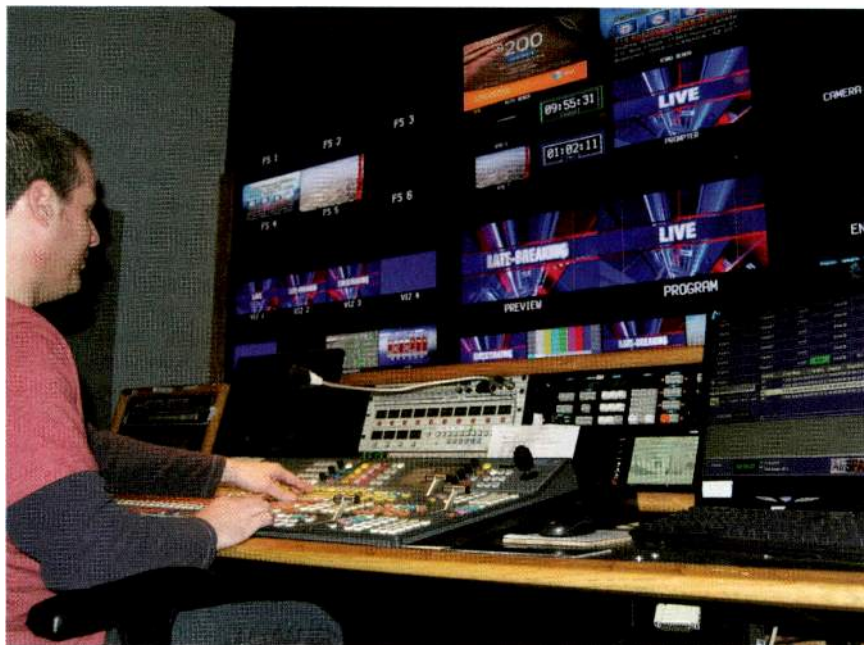
Andrew Bales, technical director for KCTV5 News serving Kansas City, MO, and KS, produces a newscast from the station’s new HD control room.
