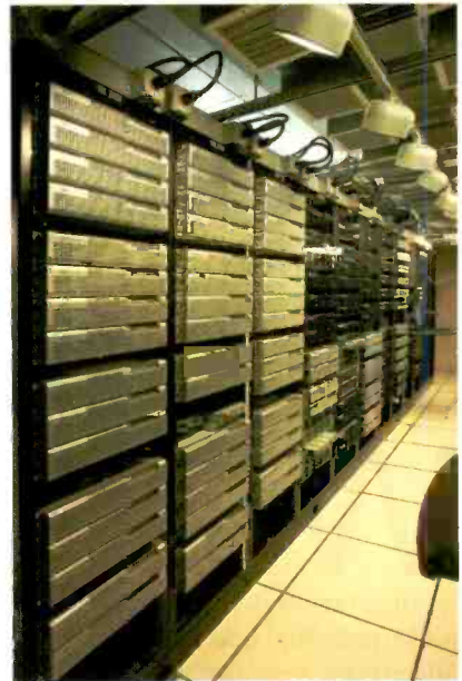
The machine room features Grass Valley K2 media servers employed in a RAID-protected SAN.
