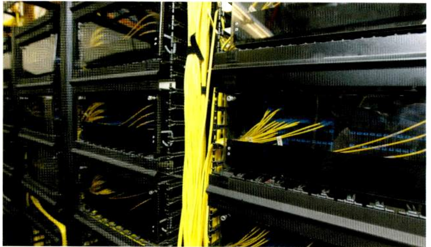
Belden FiberExpress fiber-optic distribution cables support the data backbone at Lucas Oil Stadium in Indianapolis. The main equipment room is linked with more than 50 telecommunications rooms, A/V amp rooms and other locations.
