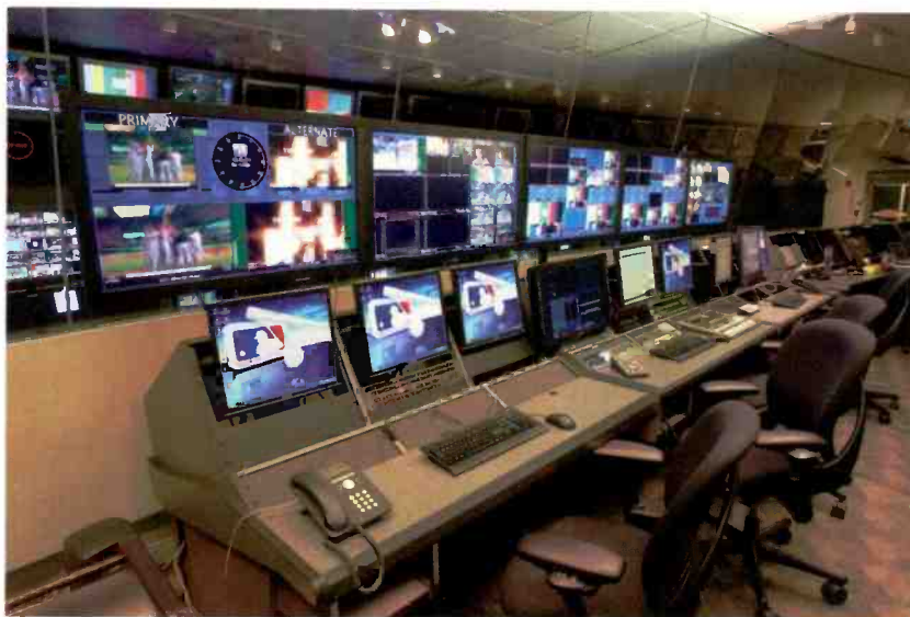
The master control area features an Evertz Quartz system, where bugs, a reality check ticker and commercials are inserted before the programs go out to air. A live ingest area with Thomson Grass Valley Aurora Ingest workstations supports QC as well as the recording of incoming satellite feeds.
