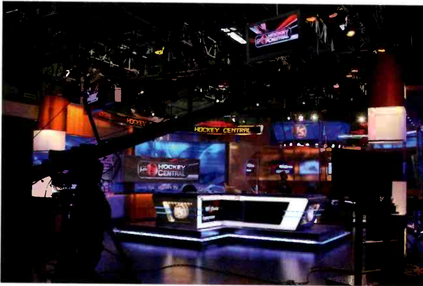
By building a free-standing aluminum truss system, Versus was able to erect a lighting grid without making major modifications to the building.
