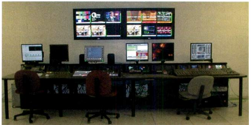
WNIN-TV, a PBS station in Evansville, IN, replaced all of its legacy analog equipment and streamlined its workflow with a complete master control and monitoring upgrade. The upgrade includes multiple screens displaying multiple outputs from a Miranda Kaleido-K2 multi-image processor.
