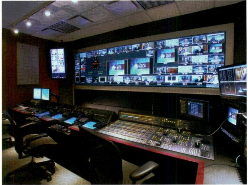
The new WETA HD video control room for "The NewsHour with Jim Lehrer" features a Sony MVS8000A switcher, expanded Thomson Grass Valley HD routers and a Barco multiple rear-projection display wall.
