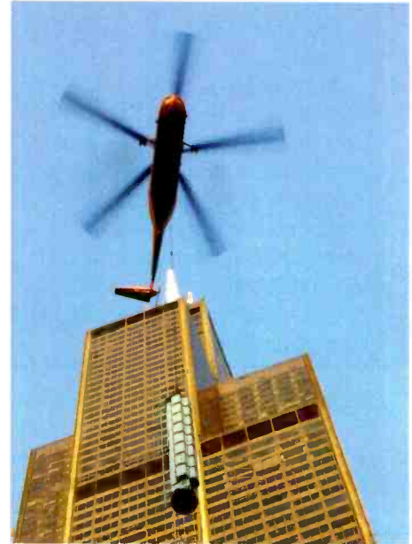
A helicopter was used to lift an antenna to the top of the Sears Tower. Photo courtesy Radio Frequency Systems.
