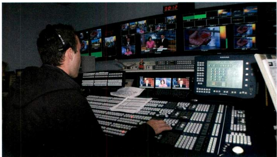
Today all is calm behind the Kahuna production switcher at WINK-TV, but a few months ago, this control room saw major demolition and rebuilding during a six-week period to upgrade to HD while maintaining control of its SD news from the room.
