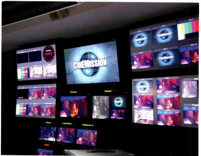
Miranda's Kaleido-X multiroom, multi-image processor was recently installed in Télé-Québec's production control area. The processor includes a router and is housed in a single, expandable chassis.
