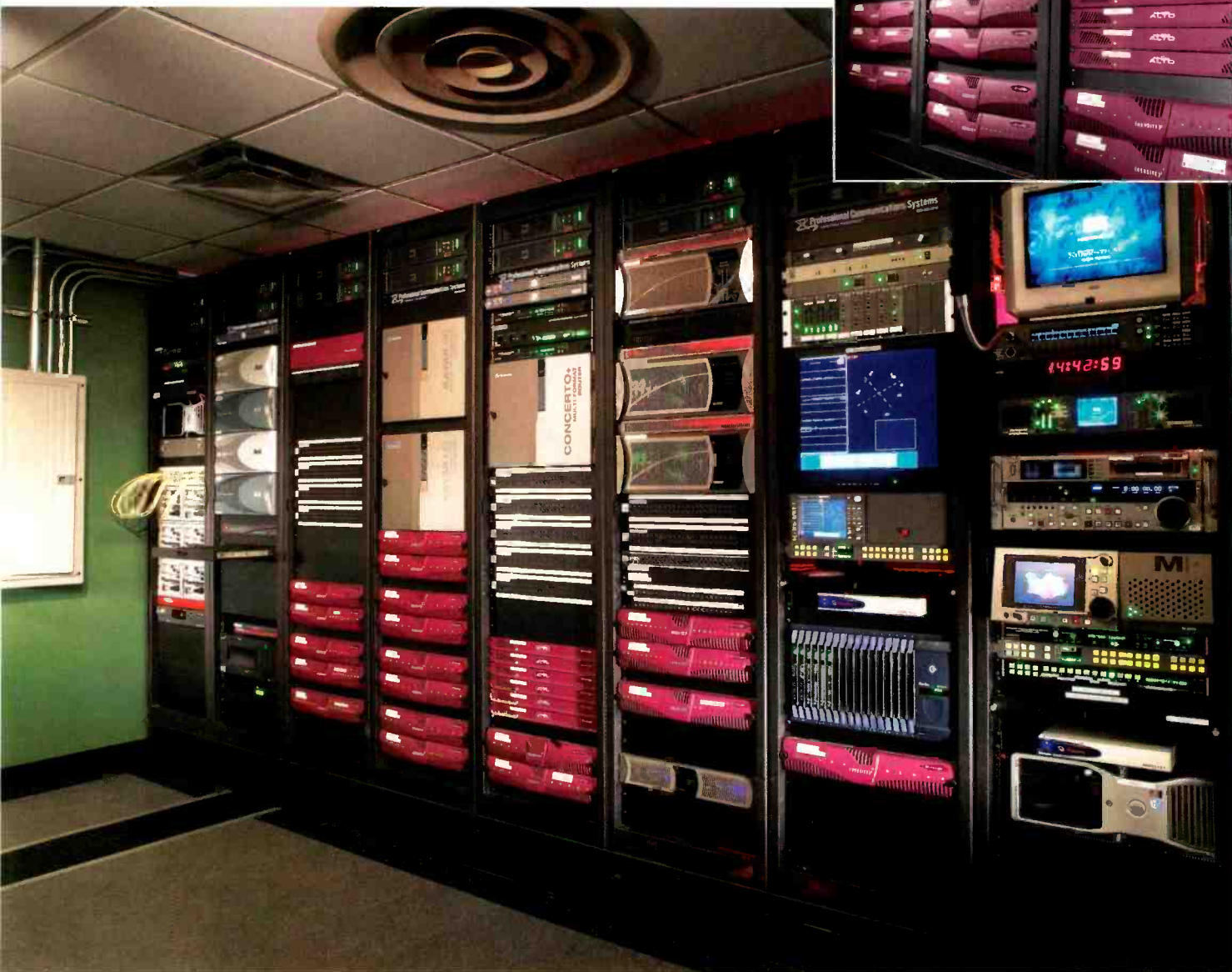
The equipment room houses most of the electronic frames in the system. The electronics frame (shown upper right) of the Clear-Com Eclipse Digital Matrix intercom system is placed on a rack in the equipment room in a secure location, separate from the two new control rooms. Also in the equipment room are Miranda Densité frames (shown middle right), containing all of the audio and video distribution, conversion, scaling, embedding/de-embedding systems and the Kaleido multi-image drivers.
