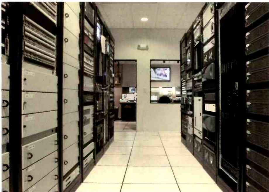
The technical operations center accommodates all the tech equipment for both the HD and SD signal flows.
