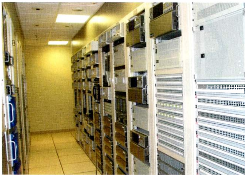
Shown here is the gear room at Turner Broadcasting Systems in Atlanta, which is monitored by the Sensaphone IMS-4000.
