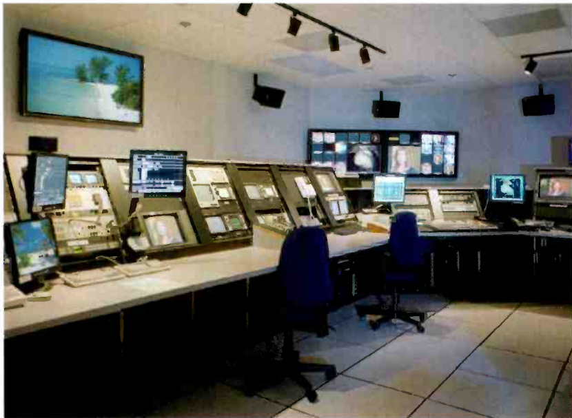
In the master control center, from left to right, are the ENG, camera control area and master control system.
