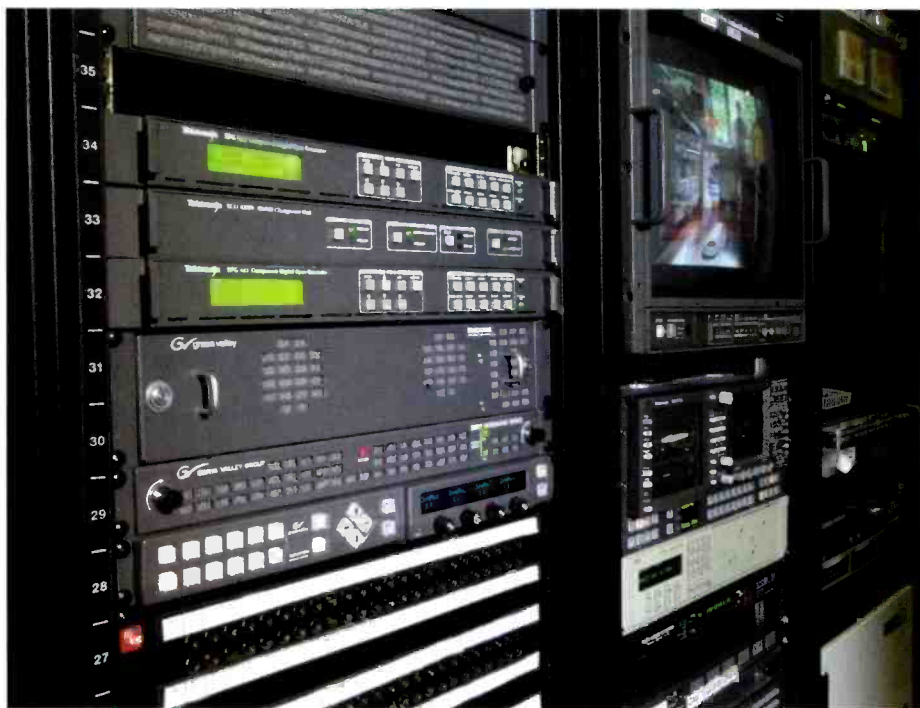
Grass Valley Encore control allows adjustment of dozens of Grass Valley components throughout the facility. The Tektronix SPG422 master sync/reference system replaced the legacy hardware. To their right is the master monitoring area.
