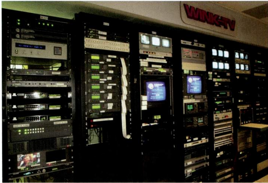
Grass Valley digital routing and conversion equipment enables the satellite control center to distribute any satellite feed to any destination in the facility.
