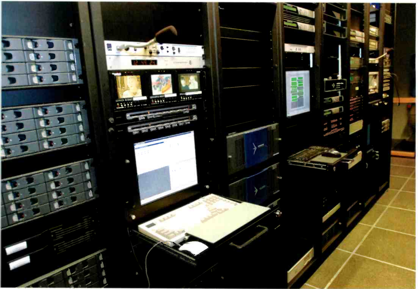
Leitch servers and Scientific Atlanta compression equipment are used in the central equipment room.
