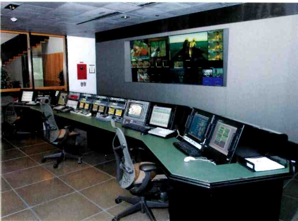
The Outdoor Channel's 24-hour master control room is situated in the facility's center with media operations and the central equipment room.
