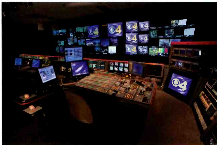
A Sony MVS-8000 switcher is the centerpiece of the technical director's position in the new production control room.
