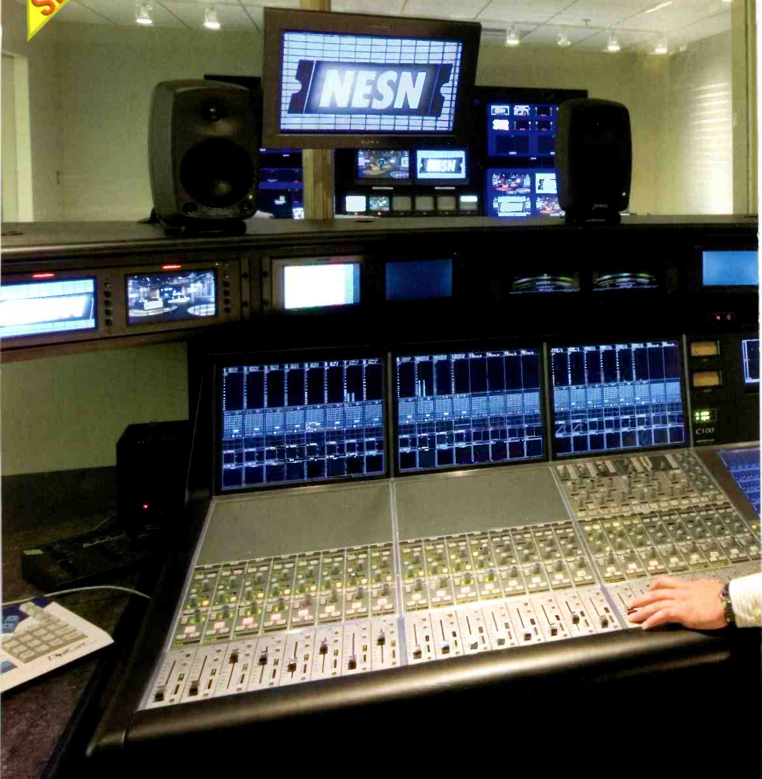
NESN's two 32-fader C100 digital broadcast consoles from Solid State Logic are at the core of a digital infrastructure that will allow multichannel audio broadcast in the future. Shown here is chief audio mixer Mike Testa at the console in Audio Control Room 1. Photos by Dave King.
