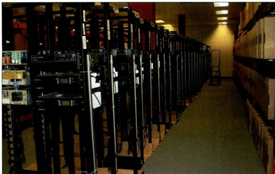
Shown here are rows of MRC DAR-2 2GHz hot-standby STL terminals, flanked by boxes of CodeRunner 2 transmitters and CodeRunner 4 receivers stored in a Sprint Nextel warehouse. Photo courtesy MRC.
