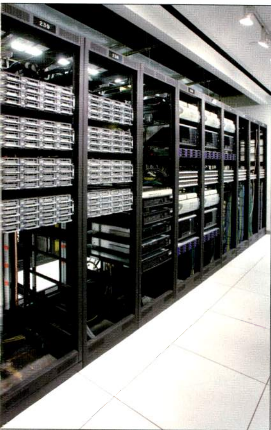
The post-production aisle in the facility's central technical area is home to Avid's Symphony Nitris and 64TB of Unity ISIS storage.
