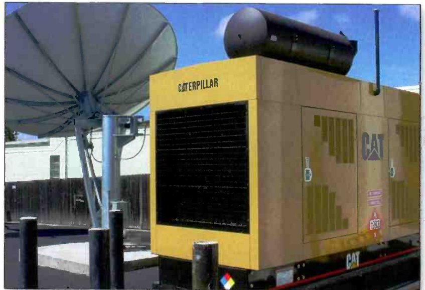
Proper integration of backup generators in broadcast operations can keep stations on the air, even under adverse conditions.
