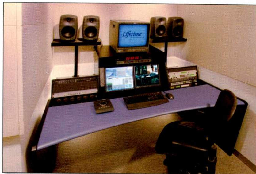
In this QC and ingest suite (one of four), real-time ingest of long-form programs is performed using an Optibase encoding system under Venaca S3 control.
