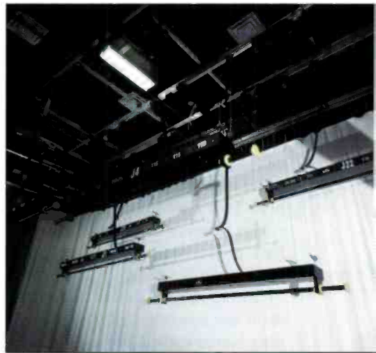
Studio A's DeSisti lighting system contains movable, self-leveling battens and an HDC hoist digital control system.
