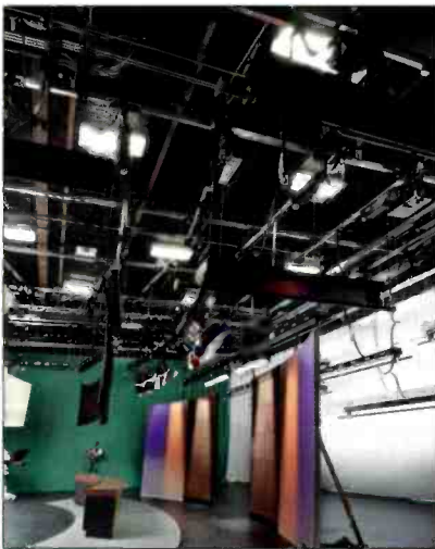
The 3800sq-ft sound stage comes complete with a DeSisti retractable lighting system equipped with 160 dimmers and HDC hoist digital control.
