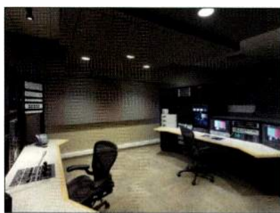
The facility's engineers provide service to the three individual stages and two control rooms from one central area. Cameras, intercom stations, tallies and routers can all be easily switched from one to another in seconds.
