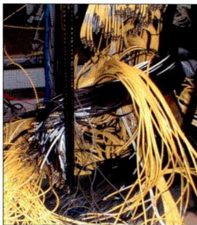
This upgrade required moving the old video wiring and starting at the beginning.
