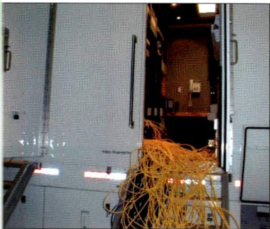
A decision must be made initially whether to save existing wiring or start from scratch.
