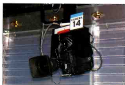
This Ikegami HDK-75EXCF camera hangs from the ceiling in Studio 1C on a dual-rail track TeleGlide.
