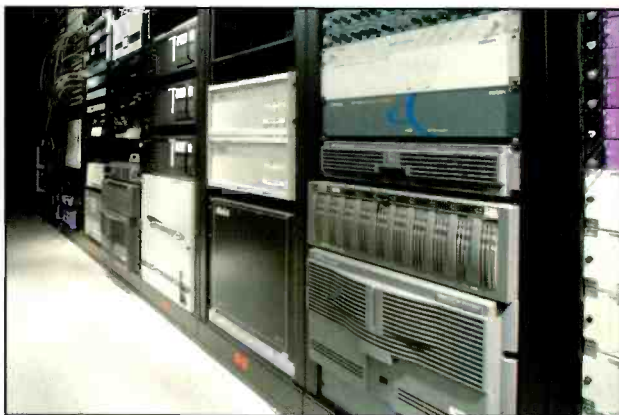
The equipment rack room features a variety of high-performance digital broadcast gear, including the Grass Valley Profile XP servers, Venus/Saturn routers, MCR switcher and Miranda processing equipment.
