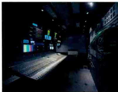
HD4's audio room features a Solid State Logic MTP digital audio console (pictured), Genelec surround sound monitors and Sennheiser mics.
