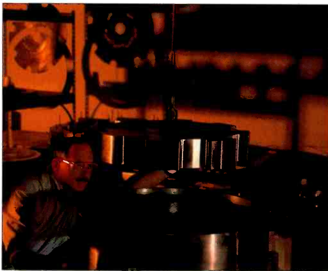
Flywheel UPS generators provide an alternative to battery-powered backups. This flywheel from Caterpillar features a 700lb. flywheel that turns at 7700 rpm.
