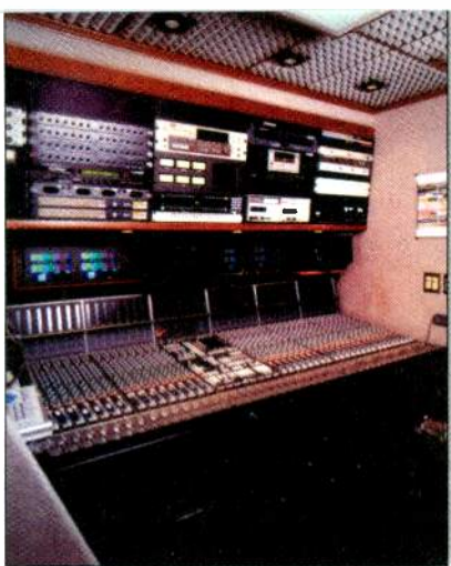
A 192-input MT Production mobile digital console from Solid State Logic is installed in Corplex's 53-foot Expando flagship truck, Sterling.
