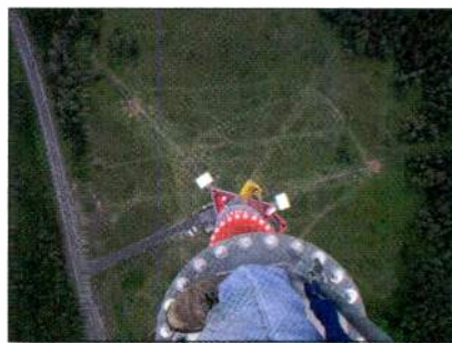
This tower-top photo was taken at the 1499 foot level of the WLEF-TV Park Falls tower during DTV-related tower strengthening.
