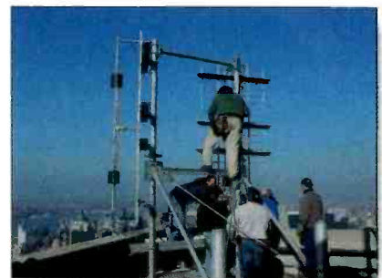
Technicians install one of two panel antennas on the 81 st floor of the Empire State Building.
