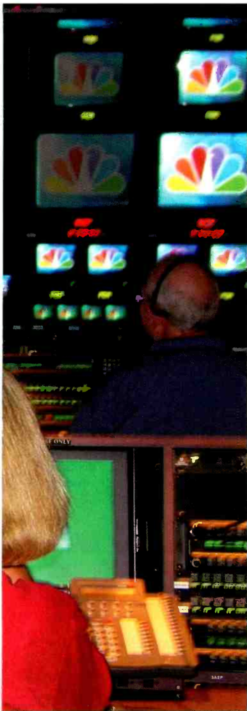
NBC's control room 3A in New York. This newsroom's communication system is fully networked with other facilities around the world through a trunked RTS/Telex system controlled by Trunk Master software. Photo by Chris Papas.
