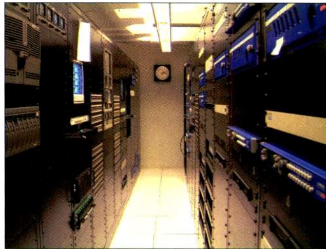
Media Most's central equipment room currently houses 32 racks of equipment, with space for 36.
