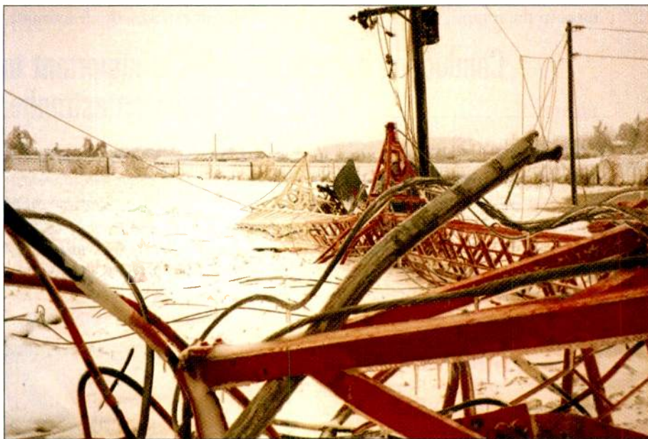
Winter storm conditions can adversely affect broadcasters. Stations in northern states may find their towers are frequently iced over, not only putting them in danger of collapses like the one shown above, but also increasing the danger of falling ice to nearby areas, cars and people.
