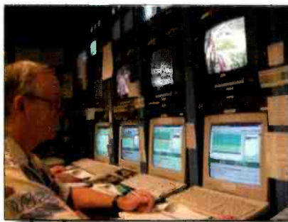
Master control operations at KGET-TV, the Ackerley Group's NBC affiliate in Bakersfield, CA. The station provides centralcasting for itself and three other stations. Photo courtesy KGET.
