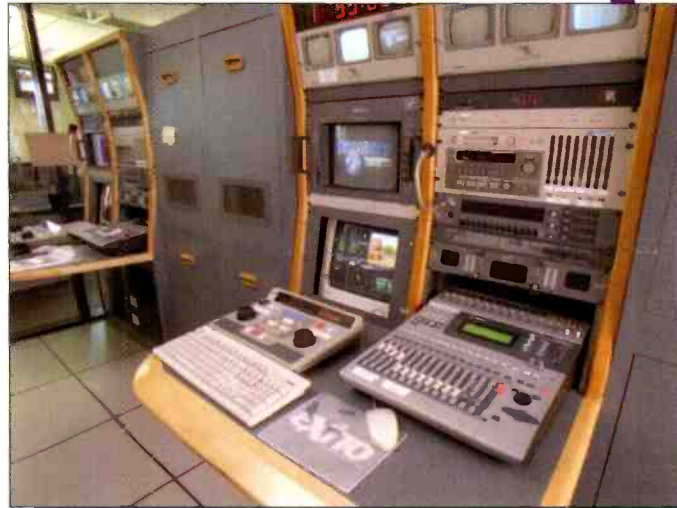
DTVC's new QC workstations are multipurpose and are used for machine-to-machine editing, screening and dubbing, as well as real-time quality control with Videotek's VTM-300, to meet increased production demands.
