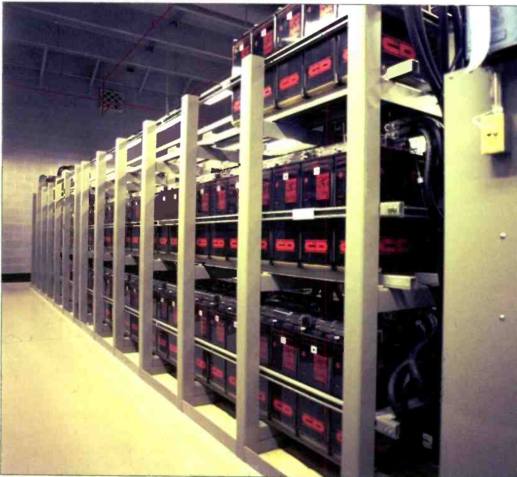
Large battery banks can serve as effective backup or can be used to assume some of the grid load during peak usage periods, a practice called peak shaving . Photo courtesy Caterpillar Inc.
