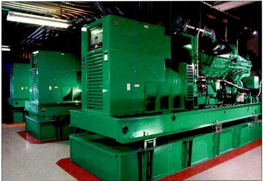
A generator should be sized to 60 percent of actual load, as loads will tend to increase over its lifetime. Proper loading will also increase its lifespan, ensuring a good return on investment.
