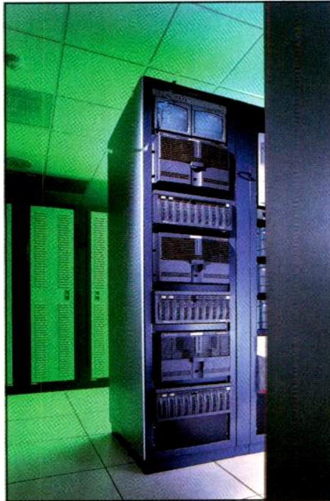
Server systems like the Grass Valley Group Profile PDR400 enable the transfer of material to editing systems via Fibre Channel, letting feeds flow directly into the newsroom and workstations. Photo courtesy Grass Valley Group.
