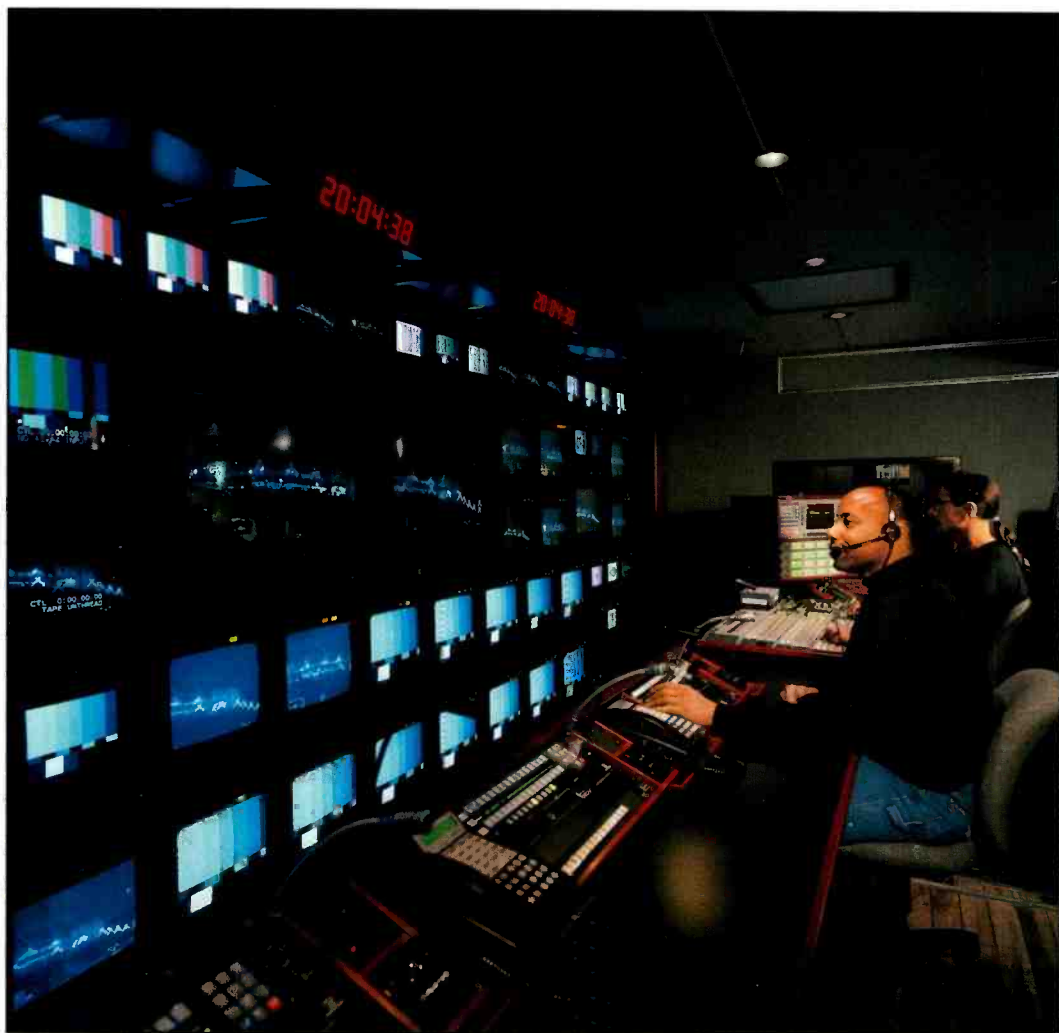
Pay attention to the sight lines of potential operators. While a seemingly small consideration, monitors at eye-level add greatly to operator comfort.
