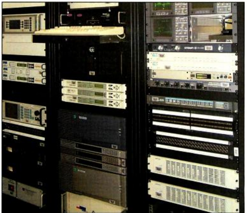
ESD 101 utilized broadband services from bitcentral to migrate to MPEG compression equipment in its uplink room, shown above.
