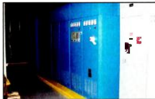
A facility-wide UPS system needn’t power everything. Focus first on critical on-air and playout systems that may fail with even a millisecond interruption in power.
