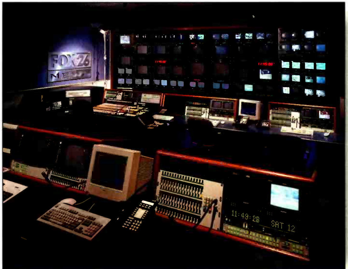
The current demands of replacing analog equipment and news branding require broadcasters to re-evaluate their facility needs. A news control room is shown here.
