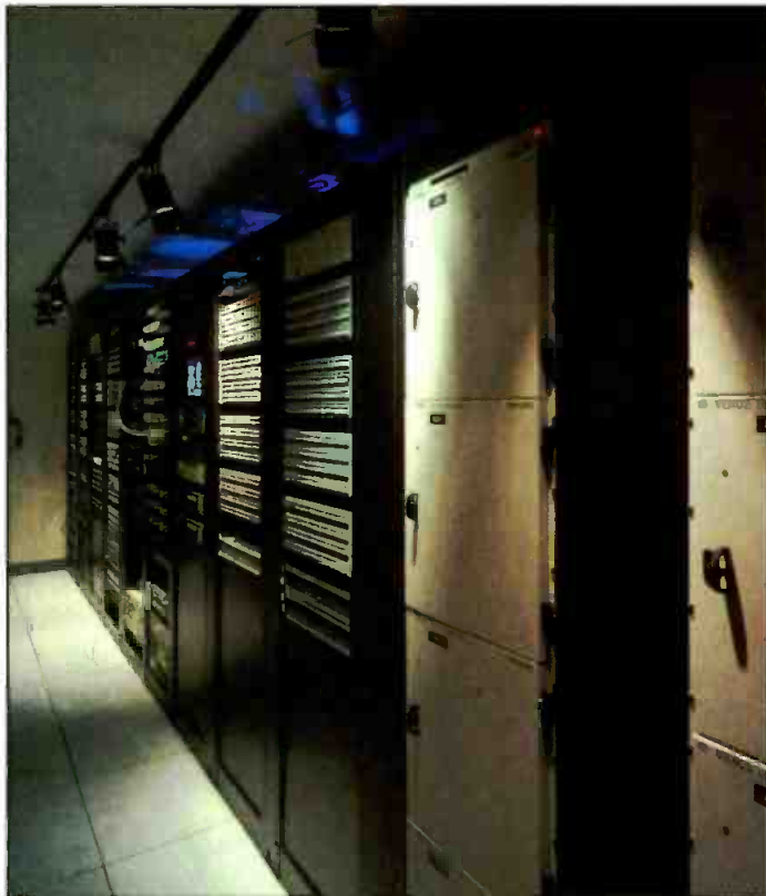
The central equipment room at XETV houses a Venus routing switcher which routes parallel video paths as one to allow easy transition between analog and digital in XETV's operations.
