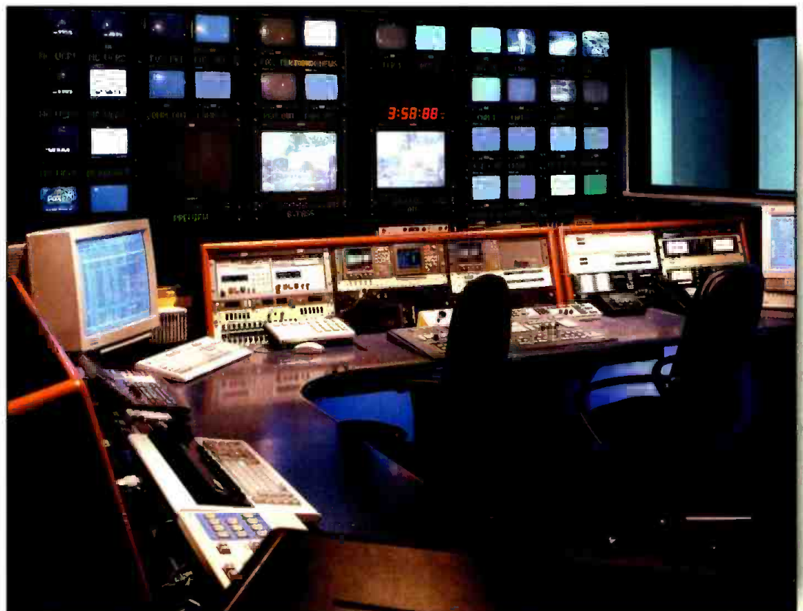
The master planning process involves determining mechanical and electrical demands for a new or renovated facility. This step requires careful thought because mechanical systems can consume up to 30 percent of a station's space. A master control room is shown here.
