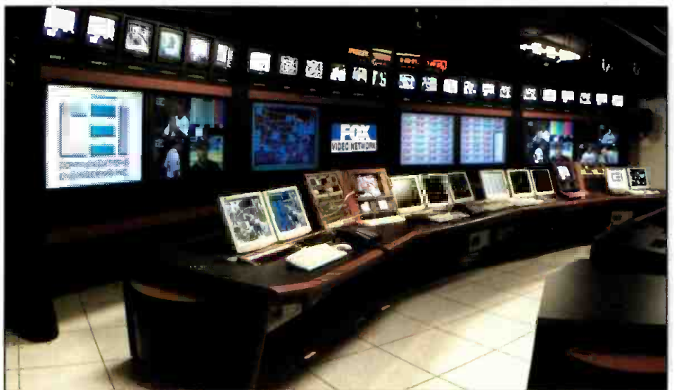
Computer-based systems make extensive use of compressed video. As computer use in facilities increases, so too will compression use.
