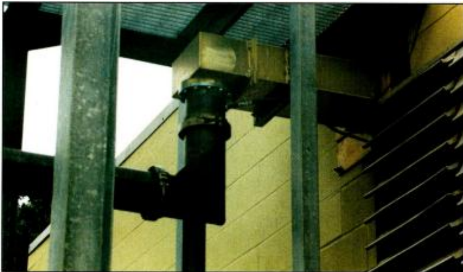
Tuning is important in systems used for multiple channels. Placing elbows too close to each other can increase the complexity of tuning the system.
