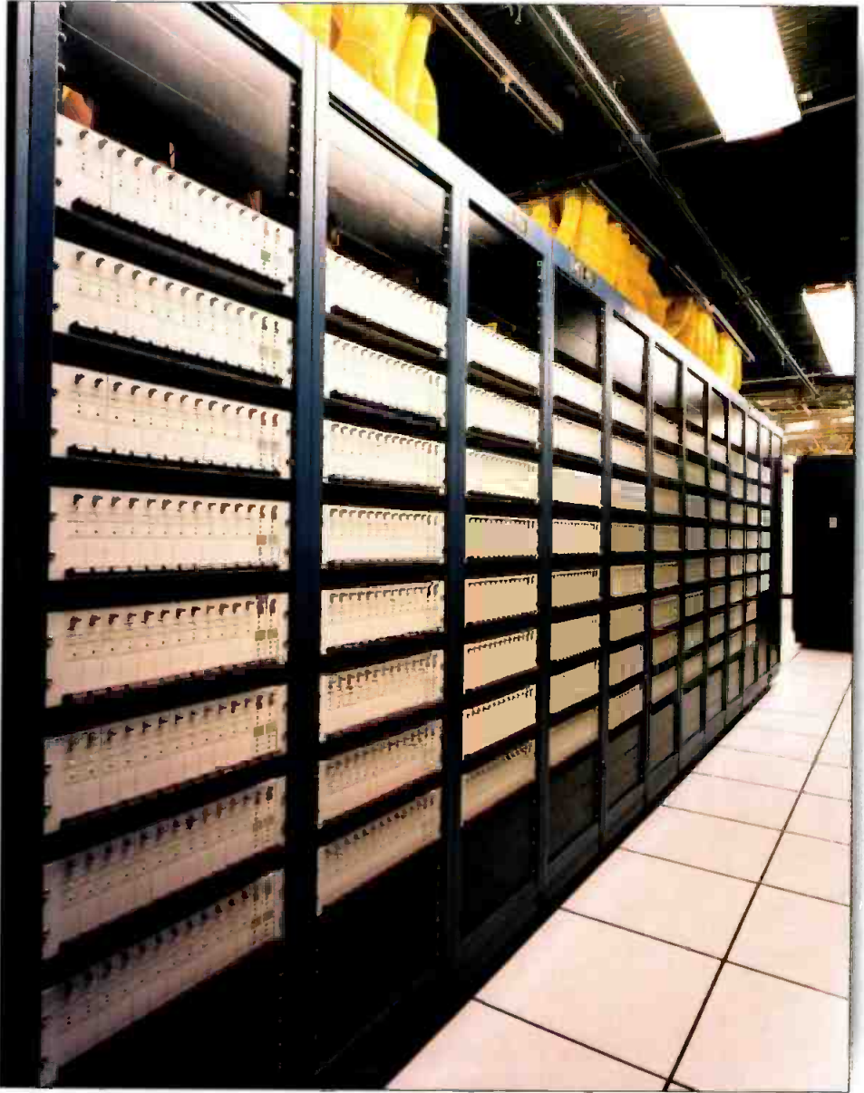
The facility's routing system employs 1024 Grass Valley Group 1x9 digital DAs feeding 32 routing frames.
