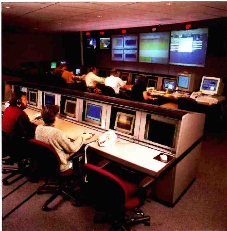
Illuminet's Network Surveillance Control Center, Overland Park, KS. Control centers such as this monitor a network of public-switched telecommunications infrastructure, helping to ensure an even spread of traffic and the highest access speeds available. Photo courtesy Illuminet.
