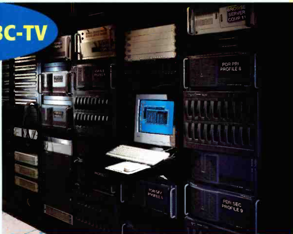
Profile video server room. A combination of Profile PDR400s, with native DVCPRO format recording and the PDR200s for on-air clips make a powerful team for the stations' fast-pace news operation. Two ingest PDR400s provide 22 hours' storage each. Material to be edited is transferred to PDR200s over Fiber Channel.
