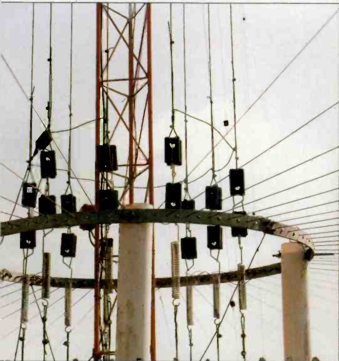
The base detail. Each fold-wire has a tension spring, two porcelain insulators and the horizontal C-ring.
