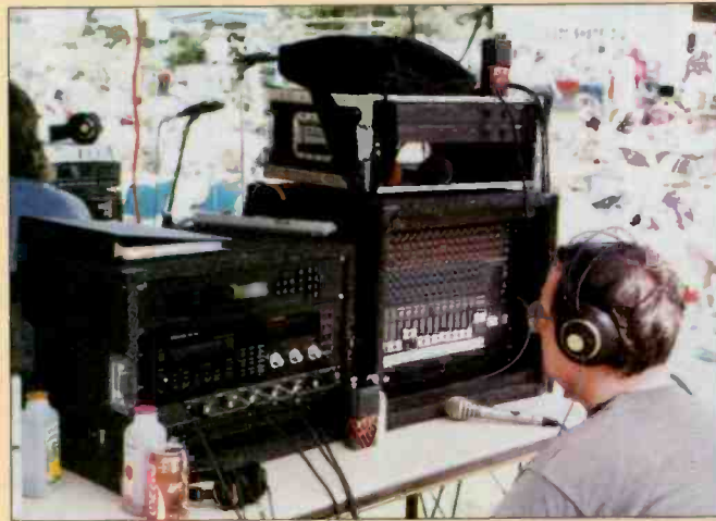
KFJC, Los Altos, CA, is a college FM station that does frequent remotes on a budget using ISDN lines for backhaul. (Photo courtesy of Mackie Designs.)
