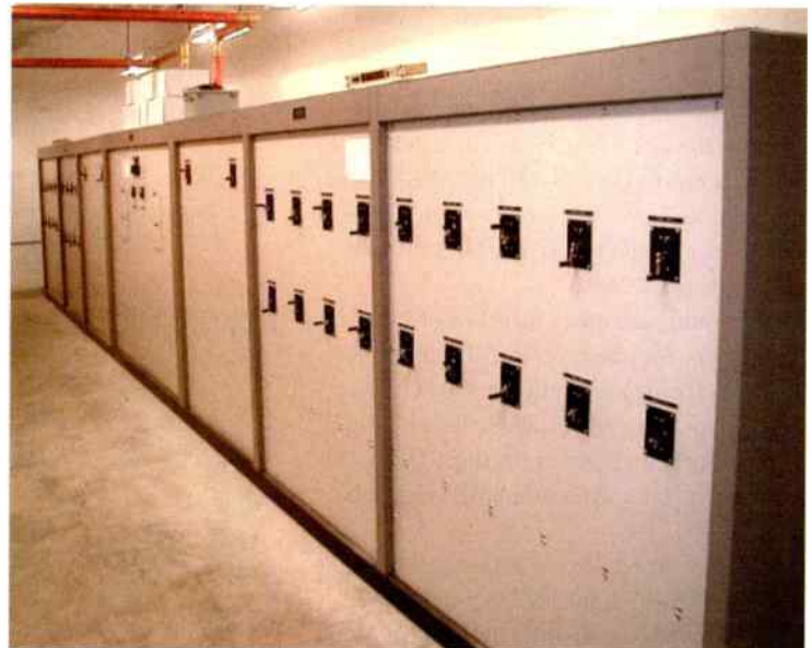
Nine-tower phasor cabinet manufactured by Phasetek.
