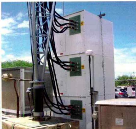
3x3 LBA "CoLoCoil" installation, as seen from the "hot" side of an AM radiator.
