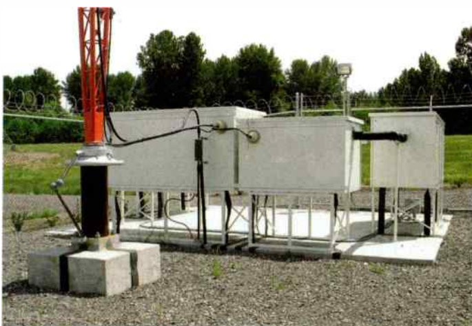
An ATU and filter combination for a diplexed system, manufactured by Kintronic Labs.
