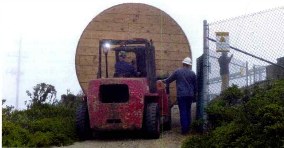
One spool of Heliac is carefully moved from the truck to a spot near the tower base.
