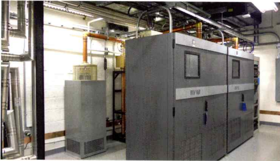
The KQED Nautel NV80 installation has a switchless combiner and aluminum hardline connections to patchfield, coaxial switches and dummy load.
