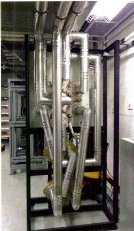
Aluminum hardline was used to connect a patchfield and two ERI coaxial switches.
