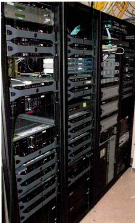
Server racks at EMF headquarters
