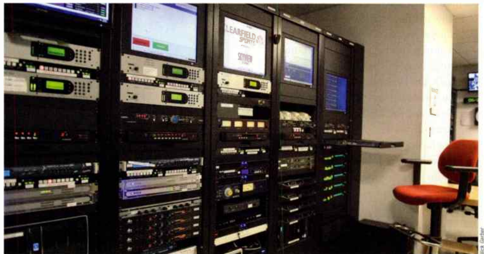
WGN rack room, featuring incoming/outgoing ISDN units, Comrex Access and WheatNet Blades.
