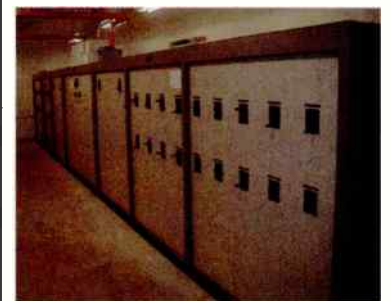
CUSTOM PHASOR INSTALLATION
