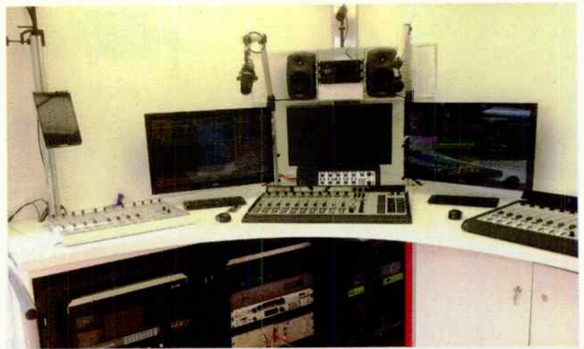
Although it is certainly compact, this set-up does not look much different than the typical stationary on-air radio broadcast studio.
