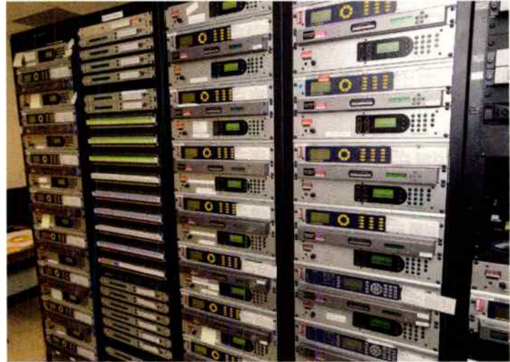
The PRSS Back-Up Network Operating Center, in St. Paul, Minn., is essential for ensuring uninterrupted service for member stations.
