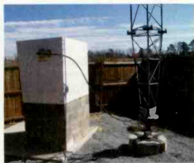
High-Power Antenna Tuning Units
