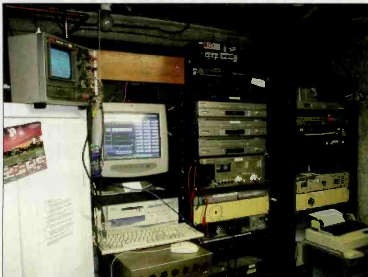
The basement is utilized as the equipment room, which made for short cable runs.
