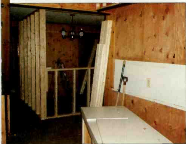
During construction, walls were built, as seen from this view from the former kitchen into the living room.
