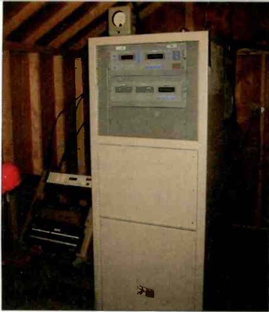
The lonely Harris transmitter with the rolling rack inside the temporary shed.
