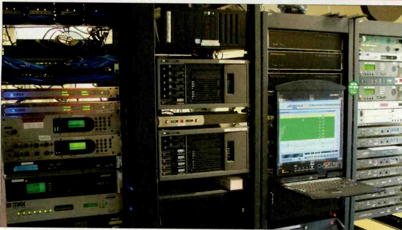
The rack room has a place for everything, and everything is in its place.
