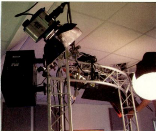
Support truss work for LCD monitors and speakers. Perfectly suited to attach T.V. lights.
