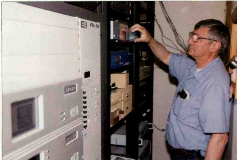
Bill Blatz in the soon-to-be-expanded RF rack room with Broadcast Electronics FMI 301 FM+HD transmitter. Adjusting one of several new Urban audio processors.
