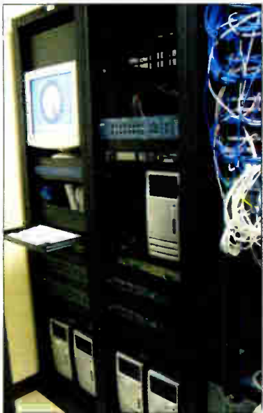
Like any facility, the rack room houses computers and computer network, and other equipment.
