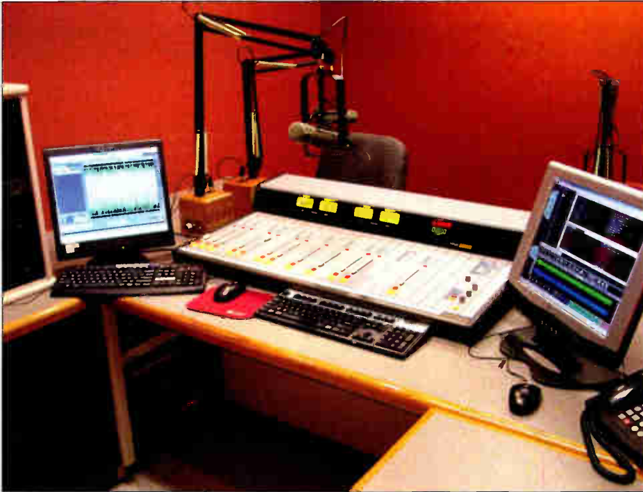
Production One, the main production studio, has a look and feel similar to the main air studios. It also has Wheatstone furniture because of its regular and sometimes heavy use.
