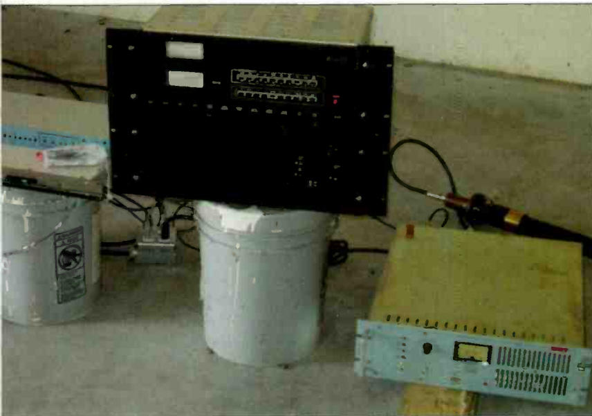
WZSP's temporary transmitter setup after its transmitter building was damaged.
