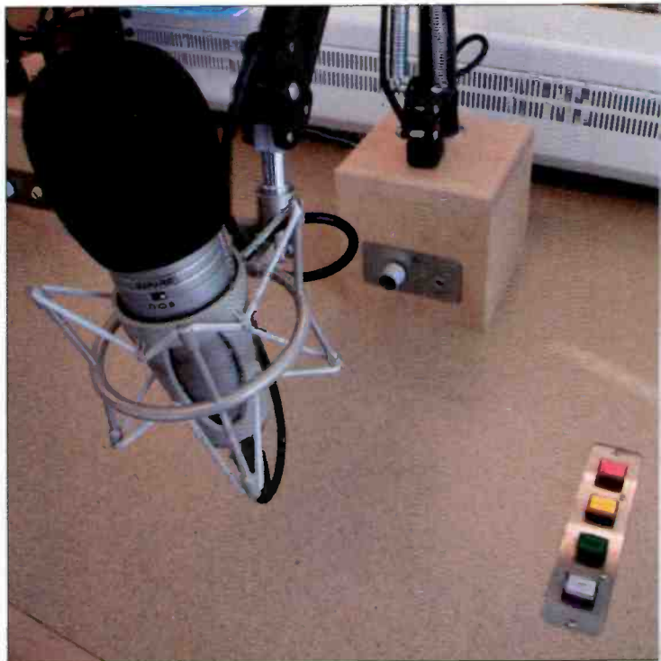
The mic booms are mounted on pedestals with headphone jacks and volume controls. Mic controls are installed on flush-mounted panels.
