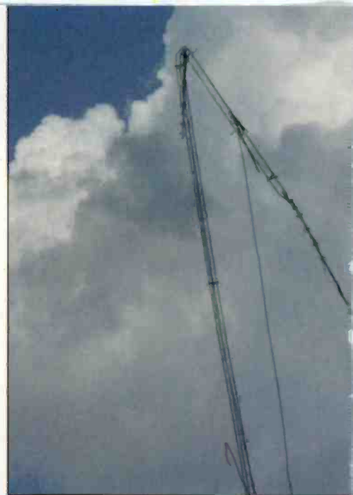
One of the more severe effects of Hurricane Charley. This tower supported two-way communications in Punta Gorda.
