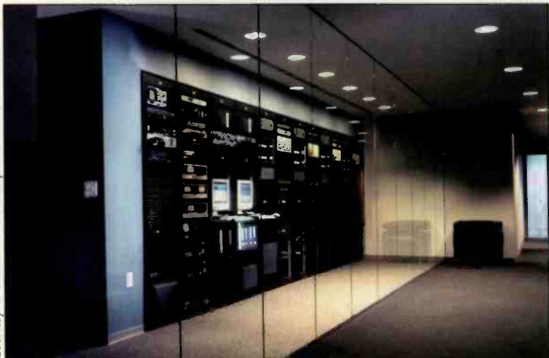
Allow enough space in the rack to provide for any future expansion, whether it is adding another station to the facility or accommodating a new format.
