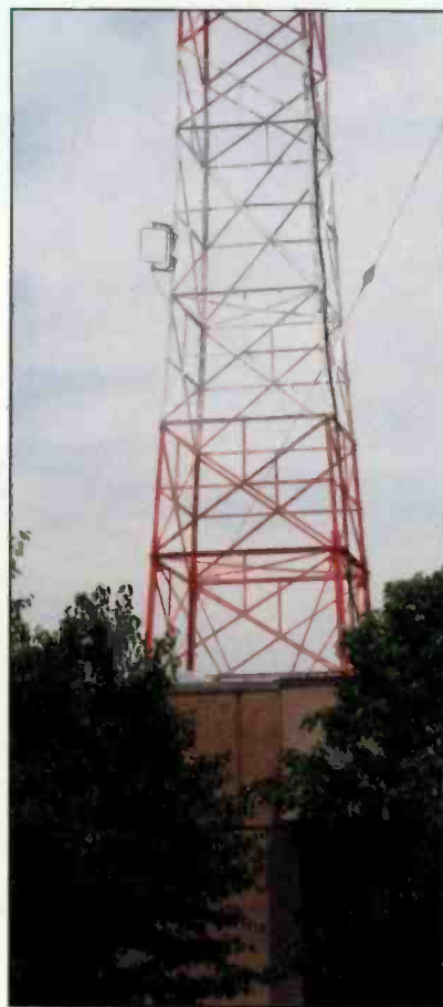
Tower-mounted pickup loops should be visually and mechanically inspected for proper orientation.
