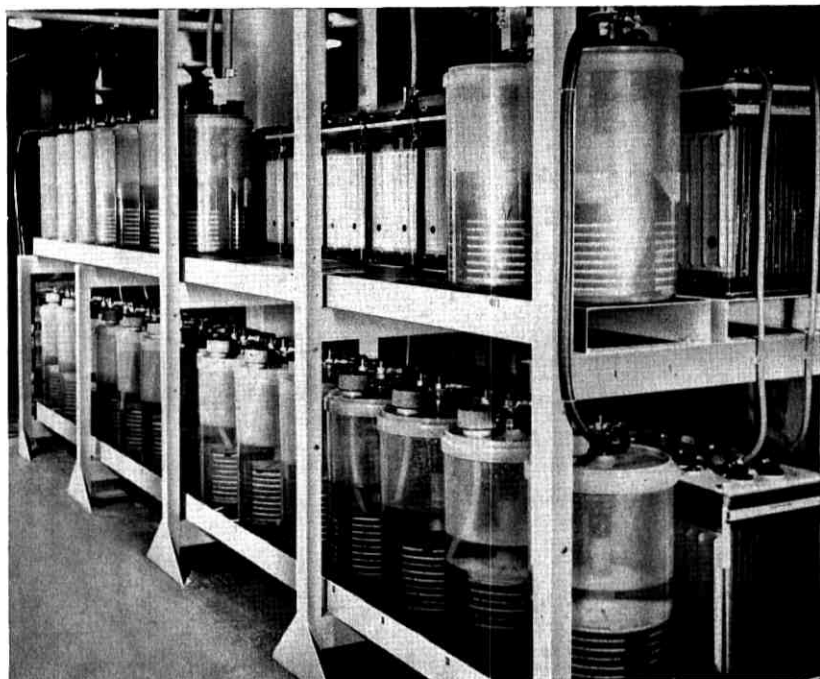
Fig. 8—Early trial installation of new cells.
