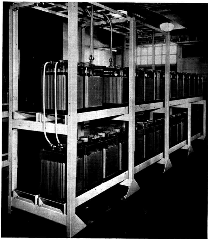
Fig. 1—Battery rack for normal service.
