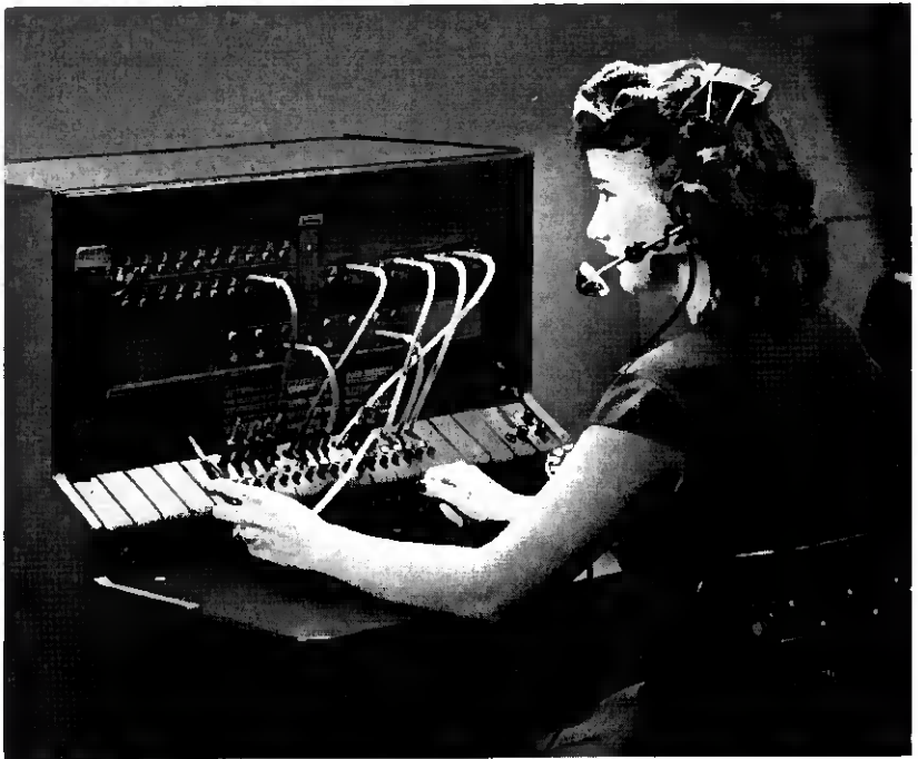
Fig. 20 — Private branch exchange switchboard, capable of handling both internal and central office calls. Used in business offices.
