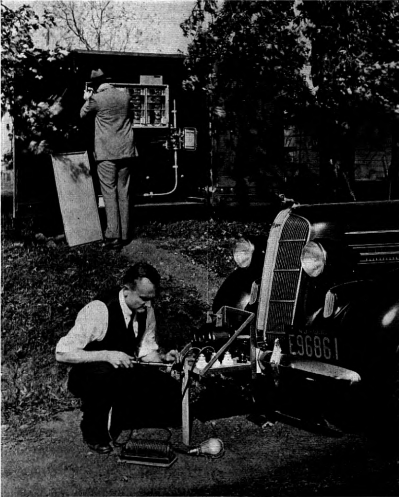
Fig. 5—Repeater near Dunellen, New Jersey.
