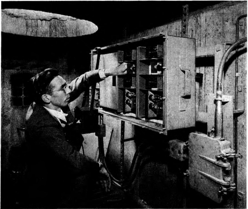
Fig. 5—Million-cycle repeater mounted in a manhole.
