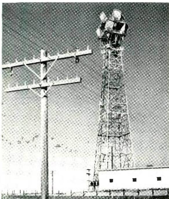
TH repeater station at Prospect Valley, Colorado. The TH equipment at this station can handle almost 11,000 two-way telephone circuits simultaneously.
